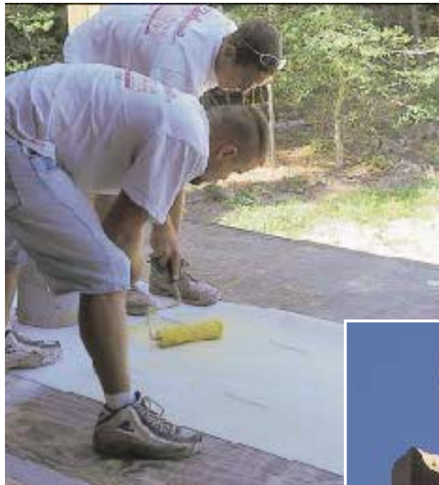
Figure 5. Beginning at the railing, the crew folds full sheets of Duradek in half lengthwise and glues the inner half to a line snapped on the deck (left). When the contact cement on the remaining half is dry, they roll the rest of the sheet into position, cutting the material to fit around posts and other penetrations (below).
