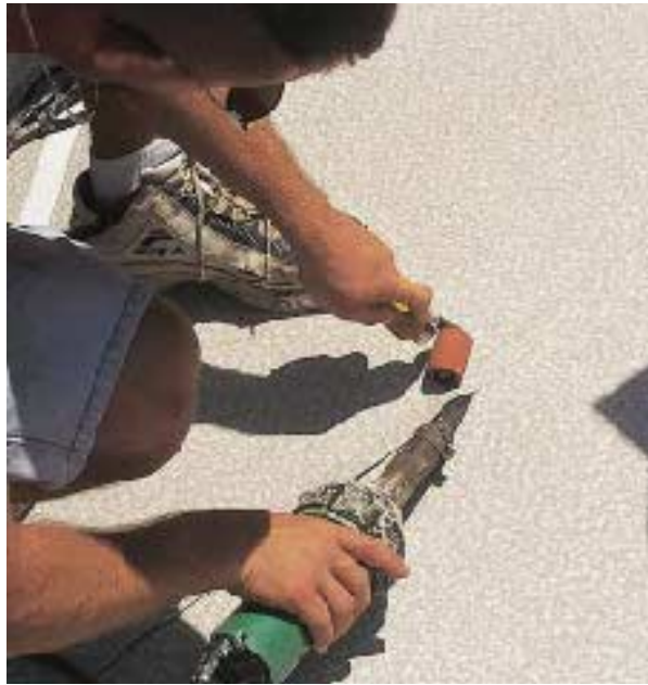
Figure 6. At the seams, the edges of the membrane are fused together using hot air from a heat gun and pressure from a hand roller (left). The same technique is used to weld flashing pieces around posts and at inside and outside corners (below).
